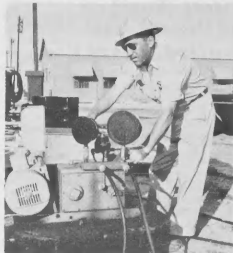
THIS HYDRAULIC pump sends fluid to the stressing jacks under pressure of 3500 pounds a square inch.
